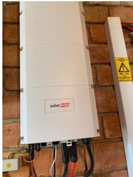
Inverter SolarEdge - RWB
